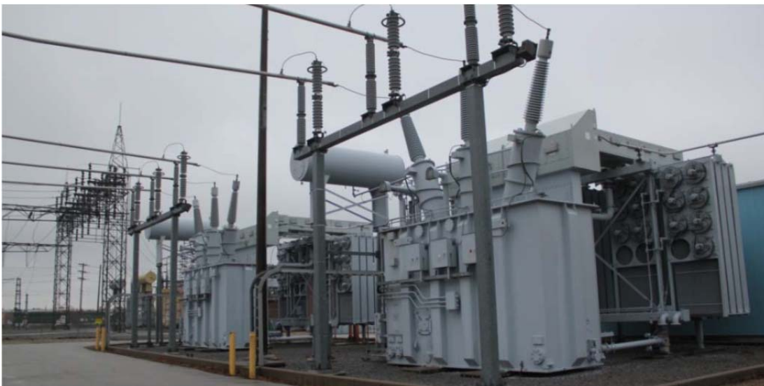
Figure 2-5 The Station Yard at Cavanagh Transmission Station
