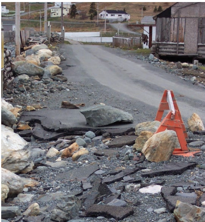
FIGURE 27: Storm-surge damage to road, April 2004, Ferryland, NL.
