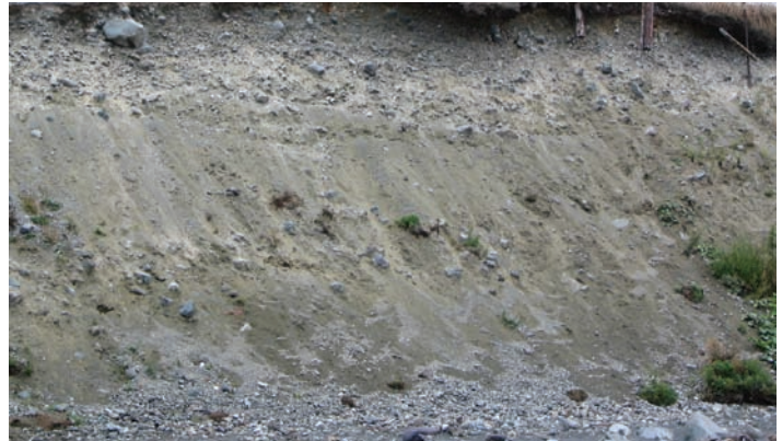
FIGURE 14: a) Coastal erosion, Union Corner Provincial Park, PE and b) Active bluff erosion, Middle Cove, NL.
